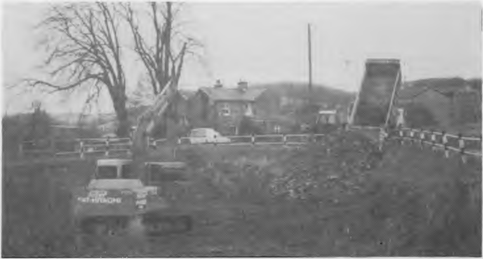
DIGGER STANDS BY AS FIRST LOAD OF CLAY ARRIVES. About 20 loads were delivered
