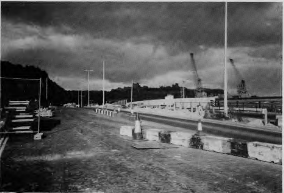
THE NEW A20 CROSSES THE RAILWAY BY THE REBUILT AND WIDENED LIMEKILN STREET BRIDGE
