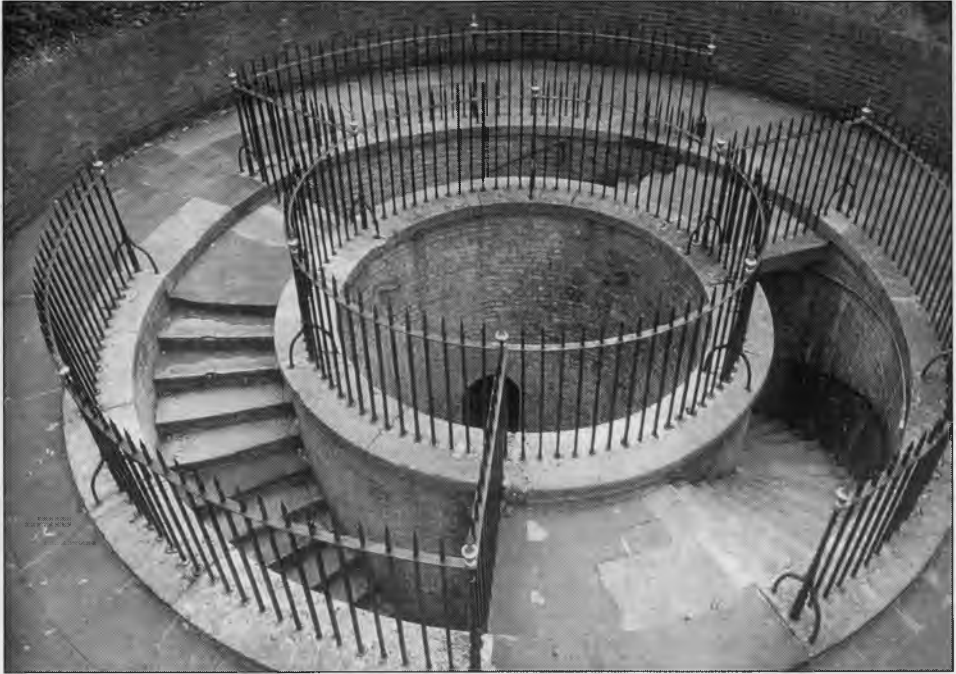
The top of the Grand Shaft showing the arrangement of three spiral staircases around a central light well.
