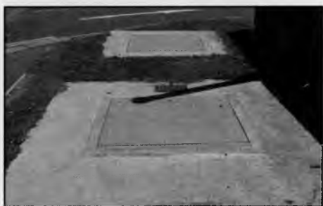
Flood prevention pumps are under the manhole covers and have recently been installed by Southern Water Limited on Maison Dieu Road.
