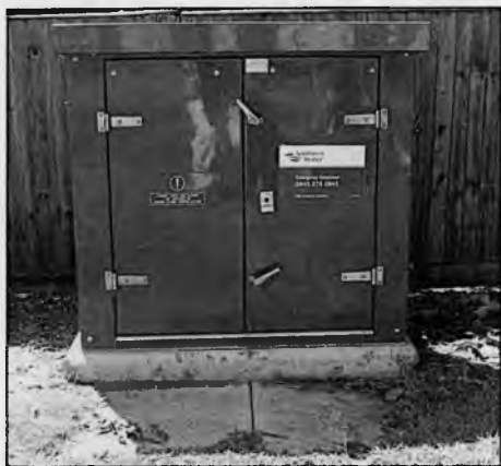
Flood Prevention Control Box Maison Dieu Road Recently Installed by Southern Water Ltd.
